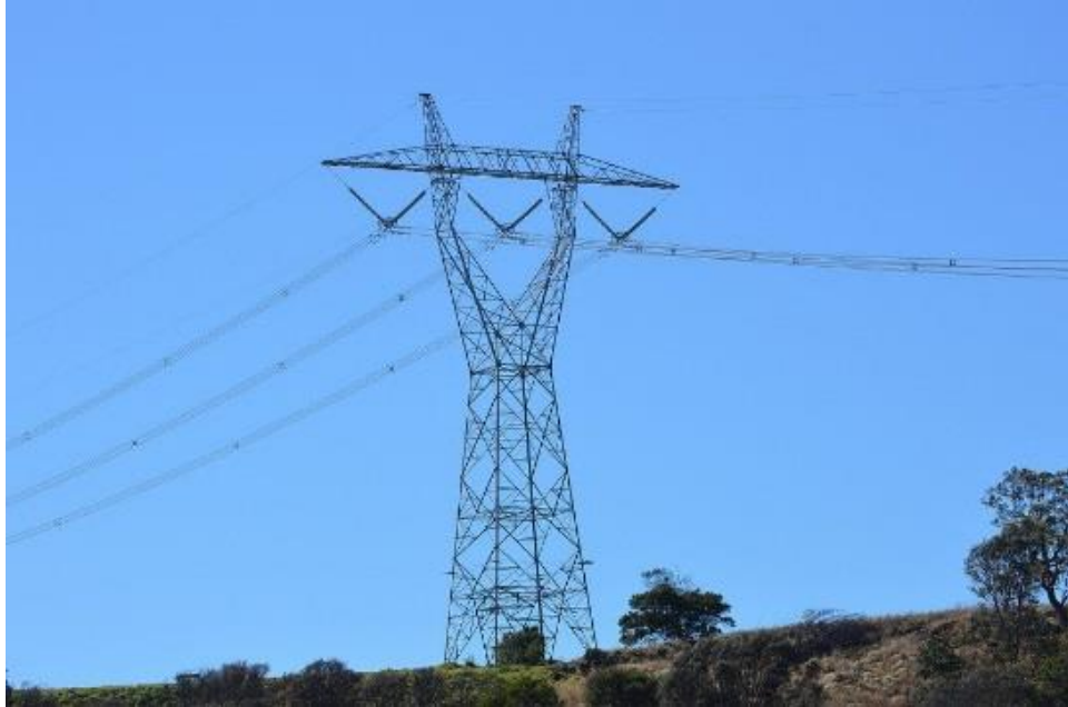
Gambar 10.3. Tower Lattice SUTET
